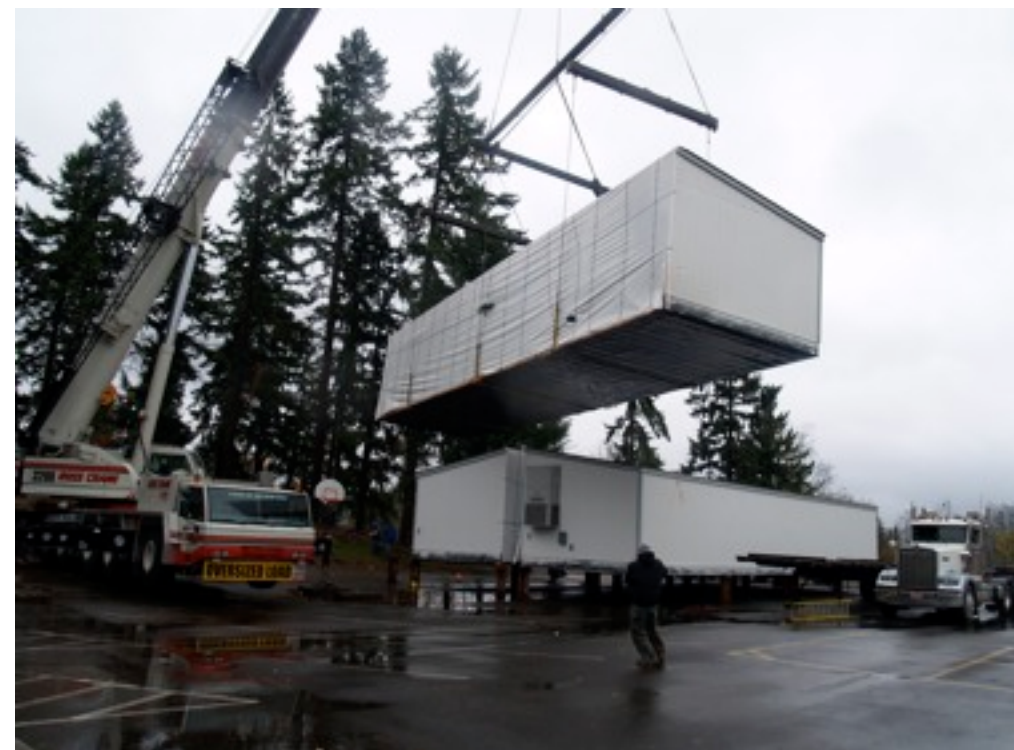
The Grace Christian High School buildings are craned into place in early November. Site work is nearing completion and occupancy is expected
